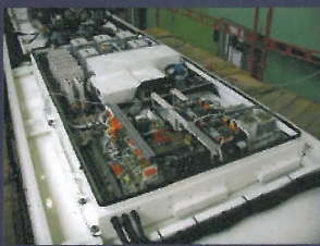
Roof container with electrical package
